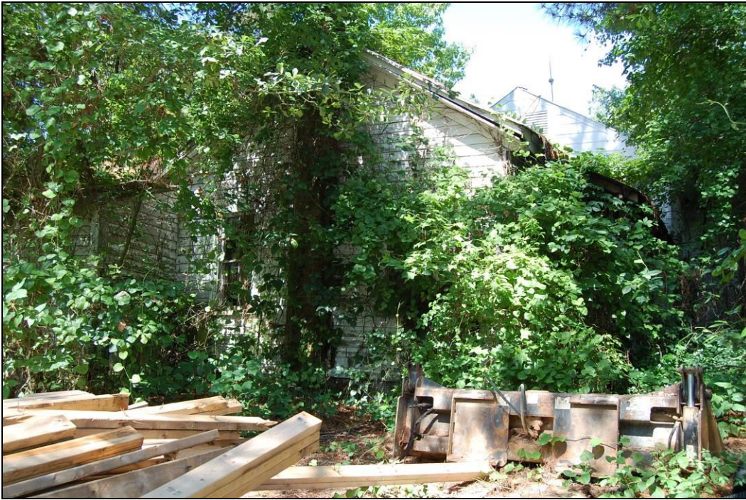
Figure 27. House, east rear elevation of kitchen wing and, at right, main block
