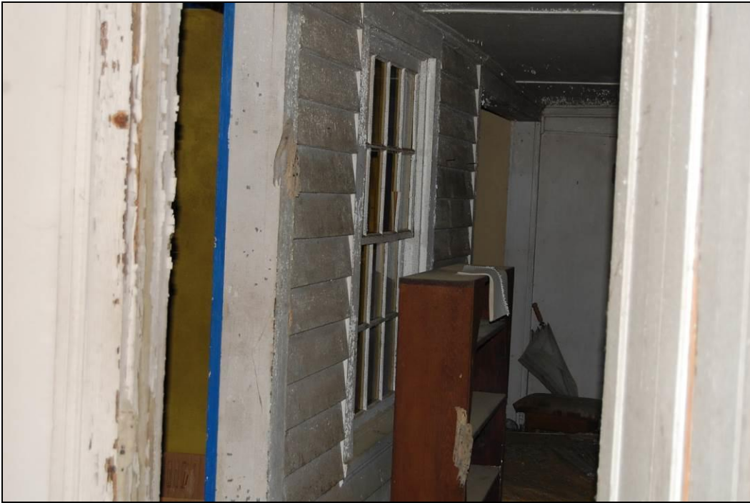
Figure 33. Looking south from central hall at former exterior wall of original rear ell; note that porch has been enclosed
